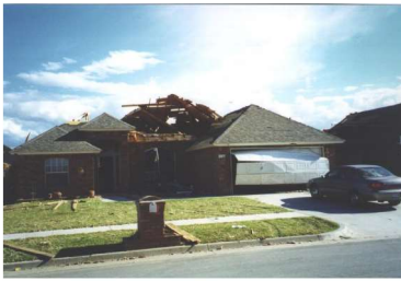
FR12: DOD 4: Uplift of roof deck and loss of roof covering (>20%); garage door collapses outward
