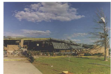
ES: DOD 9: Collapse of load-bearing walls
