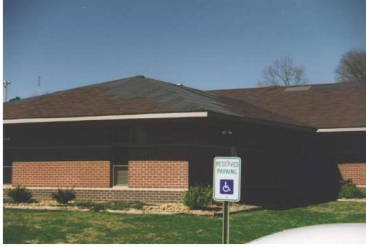
FR12: DOD 2: Loss of roof covering (<20%)
