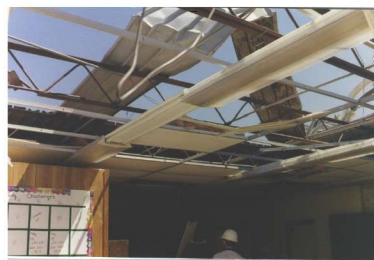
ES: DOD 5: Significant loss of roofing material (>20%); uplift of roof decking
