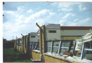
ES: DOD 8: Uplift of entire roof structure and collapse of non-bearing walls
