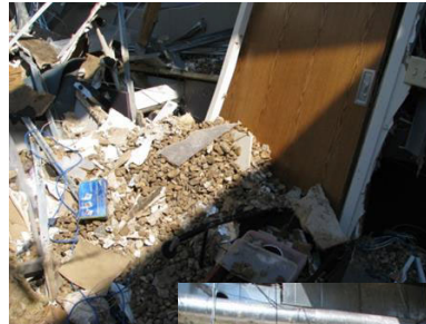
Roof aggregate inside building
