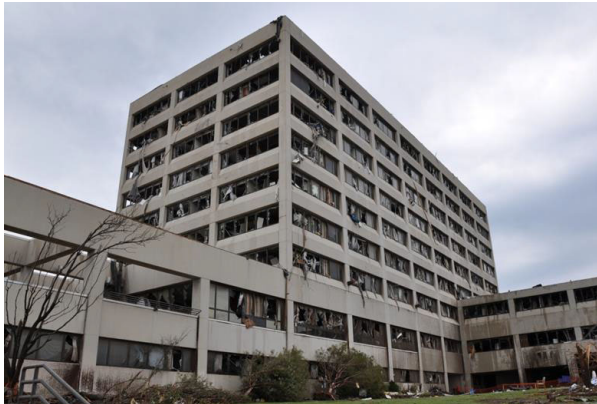
Most of the glazing destroyed
