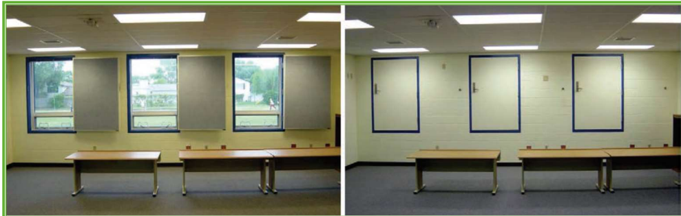
Interior operated safe room shutters in multi-purpose classroom/safe room. Image on left is normal usage; image on right shows shutters in 'lock down' position where they are closed and latched (source: FEMA P-361 3 rd ed)
